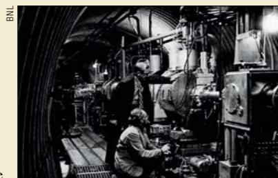
View of the superconducting magnet installed in the new beamline leading to the seven-foot bubble chamber in the North Area at the AGS.
